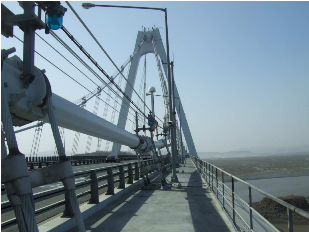
Fig. 4. Monitoring station on the cable
