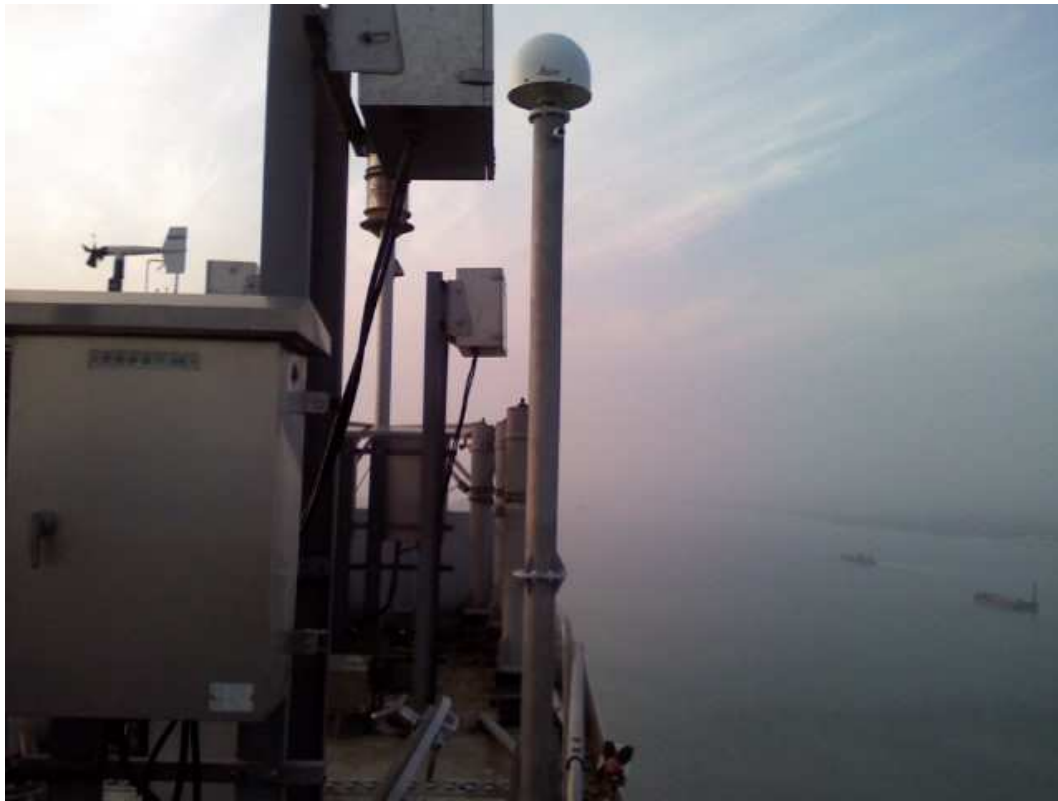
Fig. 5. Monitoring station on the top of pylon
